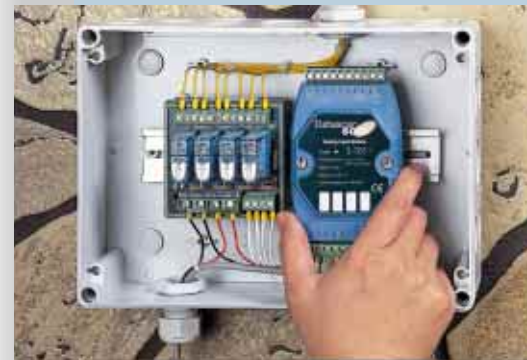
Connected to Relay Drive
